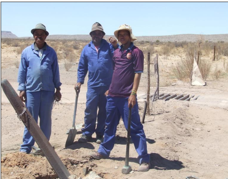
General Workers, Bobby, Josef, & Leon removing fencing prior to cattle grid removal
